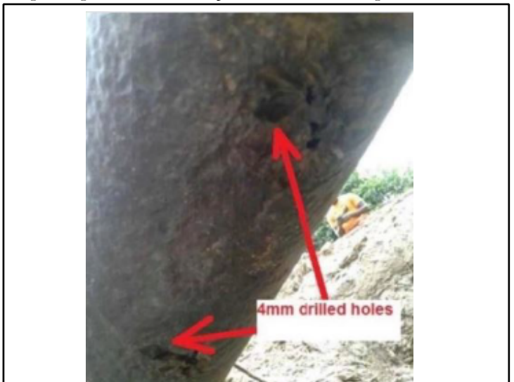
Figure 3: The holes which were identified on the pipe line was 4 mm drilled holes which are uneven and noticed that they have occurred only due to corrosion but not by human interference.
