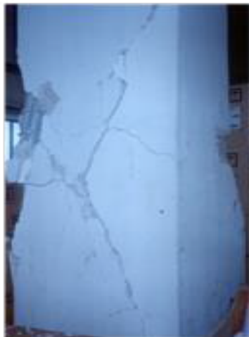
Figure 3: Column failure in Athens.
