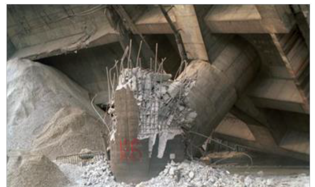
Figure 2: Pier collapse in Kobe.
