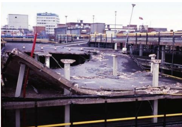
Figure 4: Car park punching.
